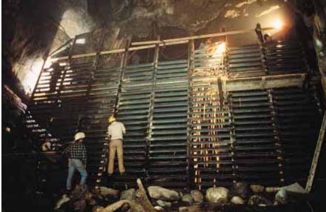
The bats of Hubbards Cave, the second most important hibernation site for endangered gray bats, were being devastated by human disturbances until huge, bat-friendly gates, shown here during installation, were erected.
